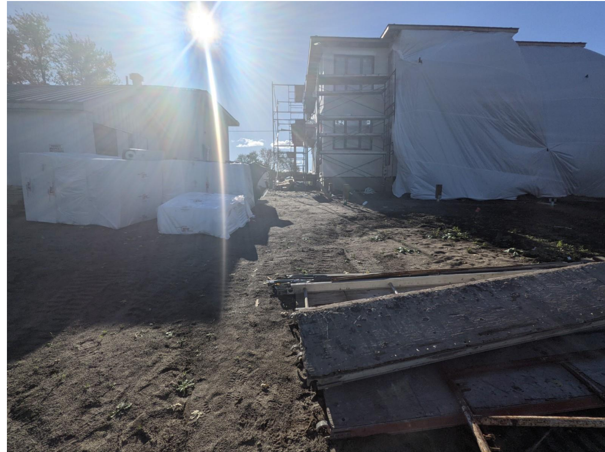
Site Photo: (taken by E. Lalande) showing area additional fill in rear yard
