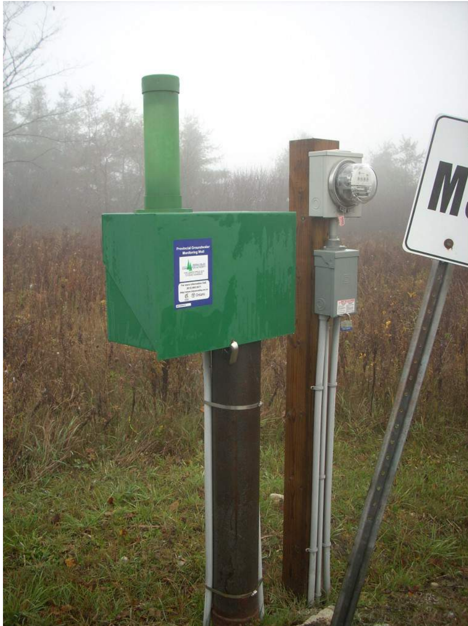
Well 83- Located in the OMYA Industrial Plant site.
