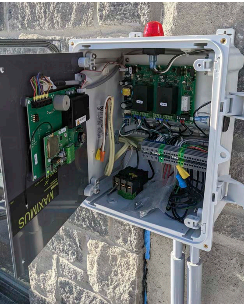
Left: Electrical control panel with red beacon alarm.
