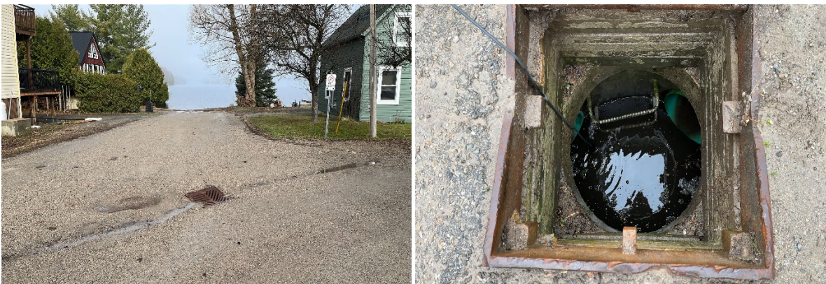
Figure 44. Exterior (left) and interior (right) view of the downstream Main & Water St. Catch Basin.
